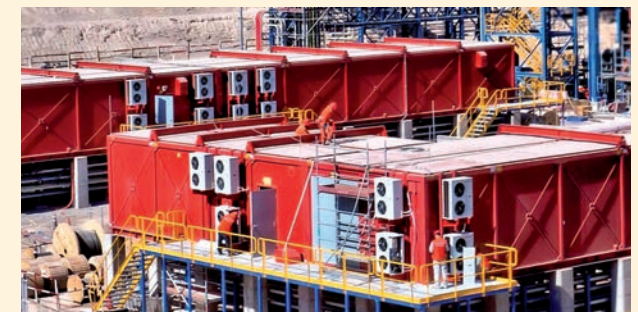
Klimatechnik HVAC systems
