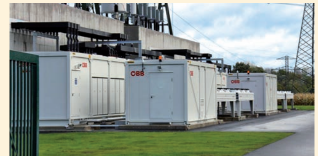
Frequenzumformstation Frequency converter station
